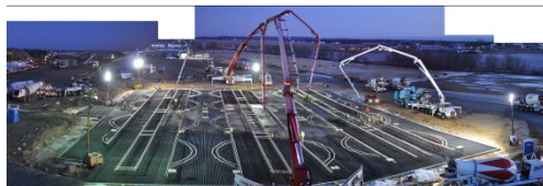
J&L provided steel and electrical services on the Chippewa Falls Sand Plant project
